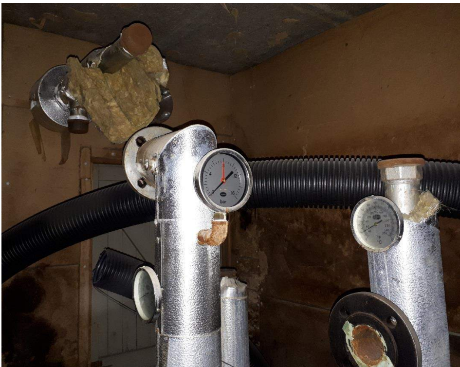
Figure 12: Disconnected distribution pipework
