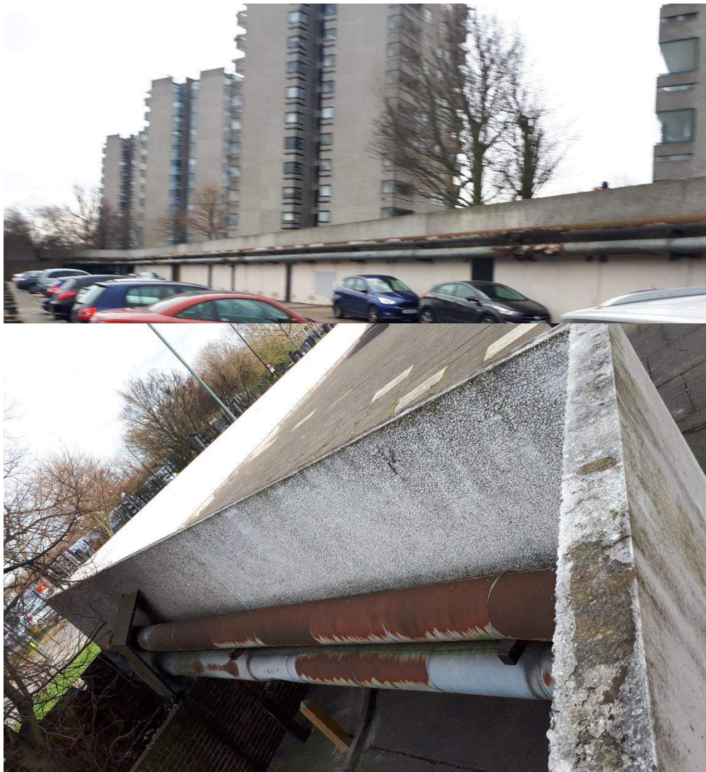
Figure 14: Examples of above-ground defunct DH pipework
