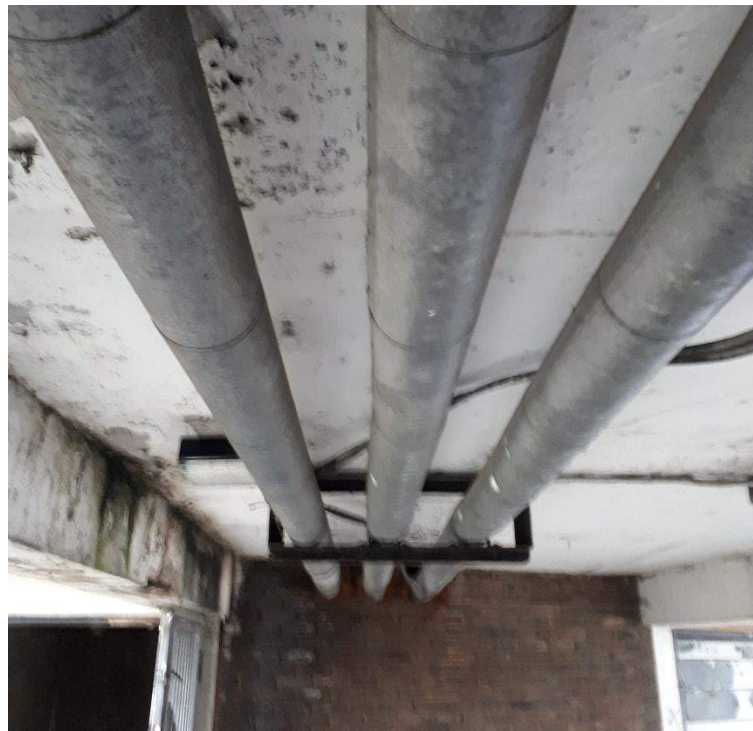
Figure 8: Defunct DH pipework running with car park area
